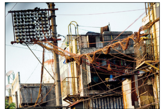
► Chaotic electricity lines are a feature of Filipino cities
