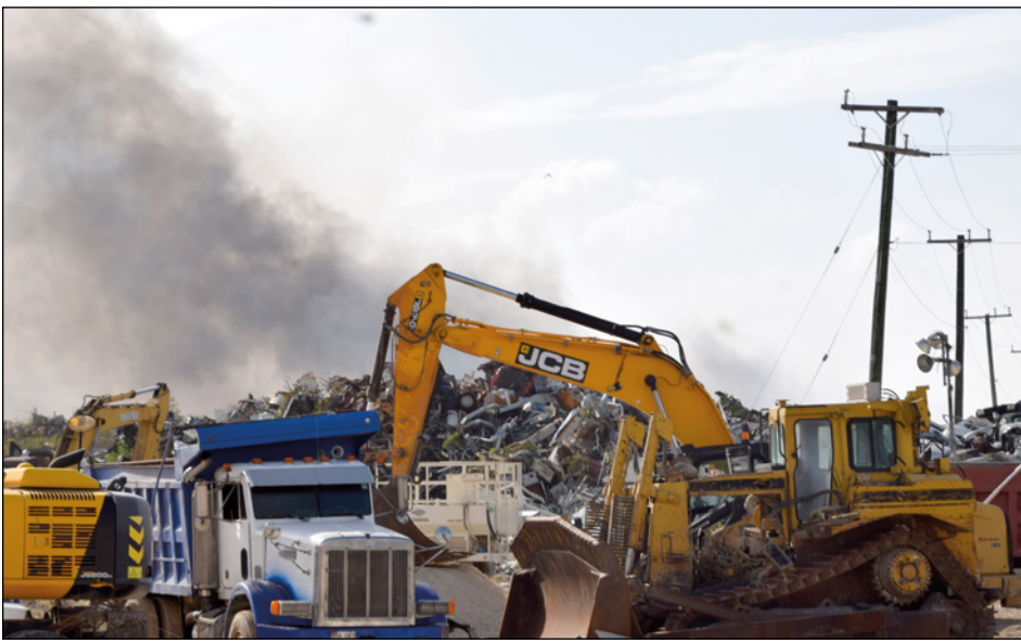
► The fire continues to burn
