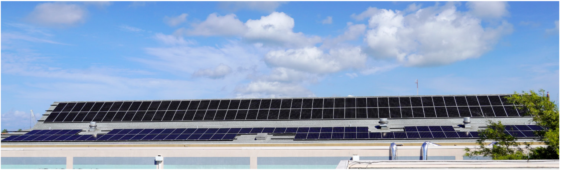
► Solar Panels completed on at the main campus of the Cayman Islands Hospital
