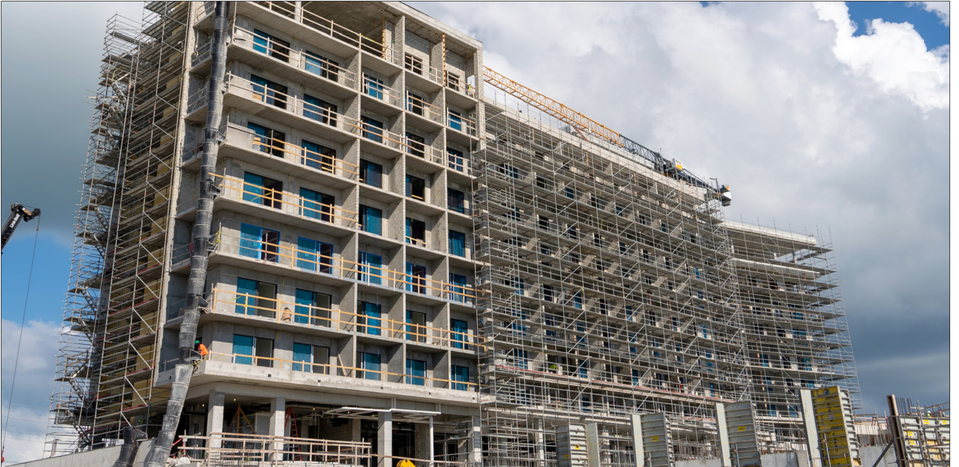
► Construction site of Hotel Indigo – Dart has been working with local subcontractors on the 282-room Hotel Indigo Grand Cayman.
