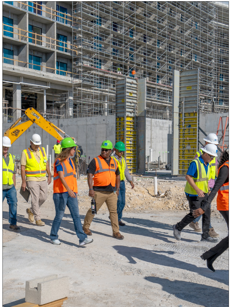
► Members of the Dart construction team and Chief Officer Wesley Howell, Ministry for Border Control and Labour, during a walkthrough of the Hotel Indigo construction site.
